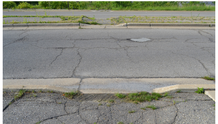
Sidewalks and pedestrian crosswalks are deteriorated
